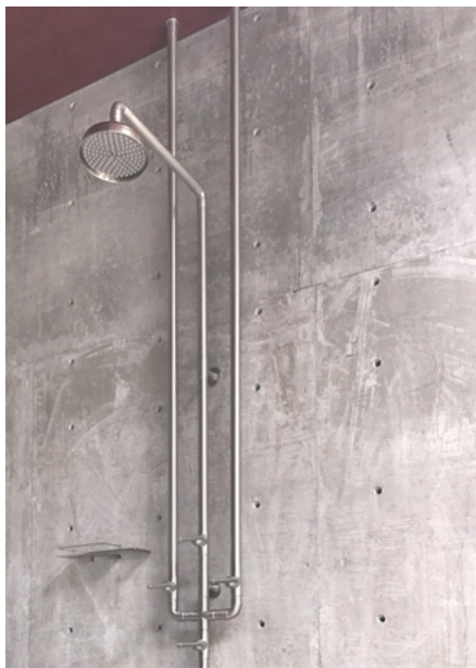
Custom swimming pool shower with ceiling mount water supply.
